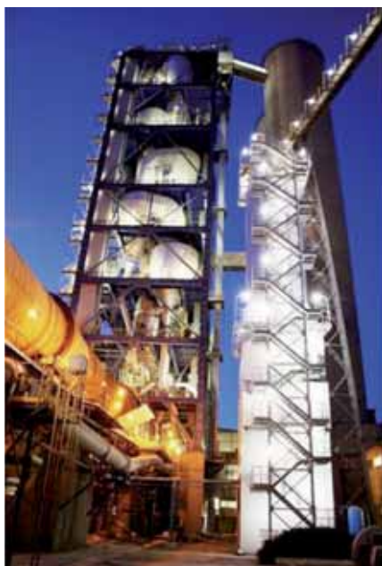
As part of the extensive upgrade, the plant's pyroprocessing stage received a new five-stage preheater tower
